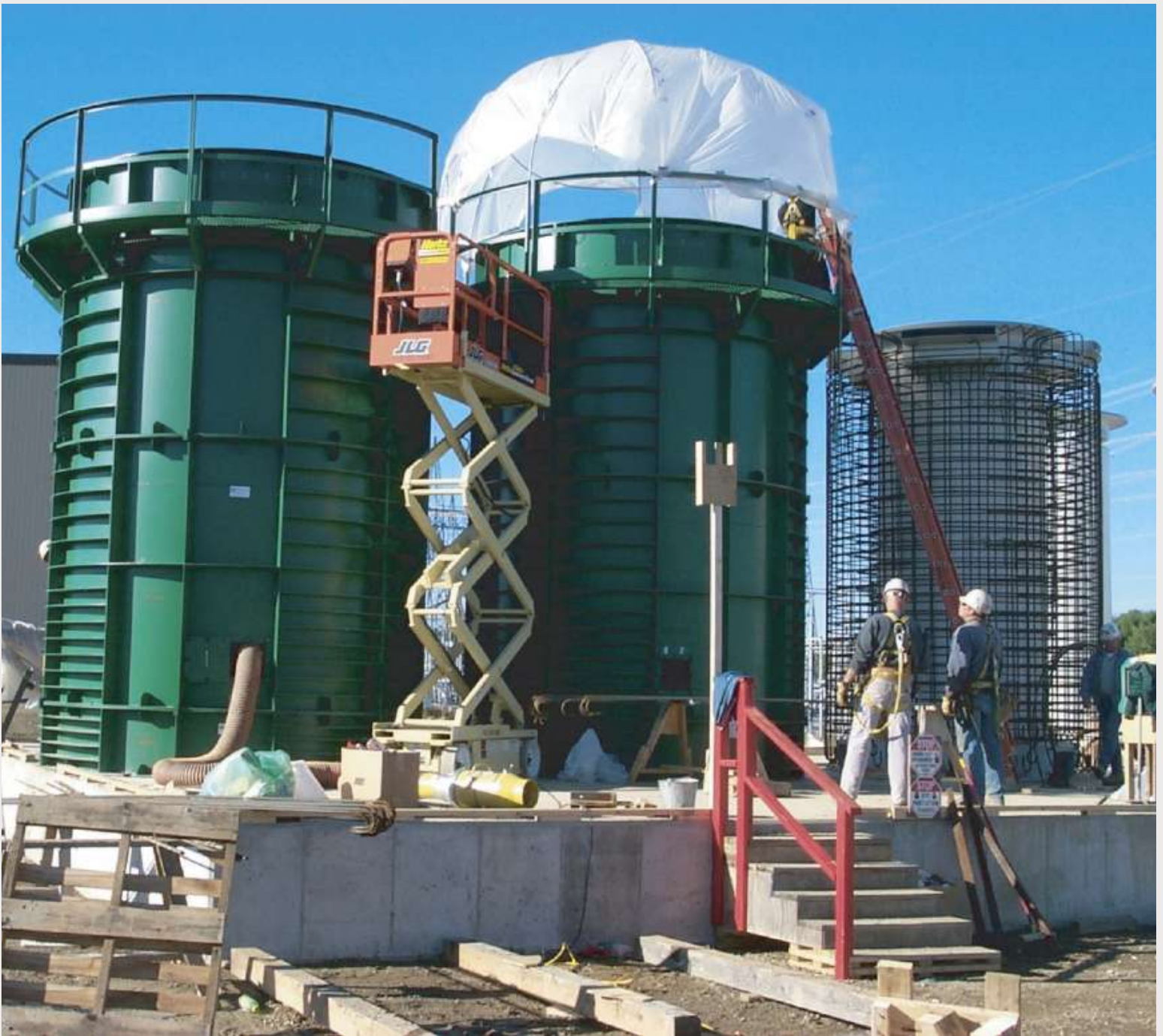
NAC dry cask storage facilities for spent fuel under construction at Maine Yankee nuclear power plant.
