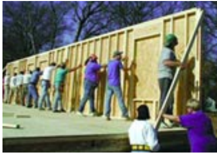
USEC employees at work on a community project—building a Habitat for Humanity house in Paducah.
